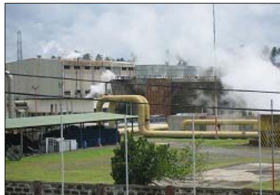
Mak-ban Geothermal Power Plant
