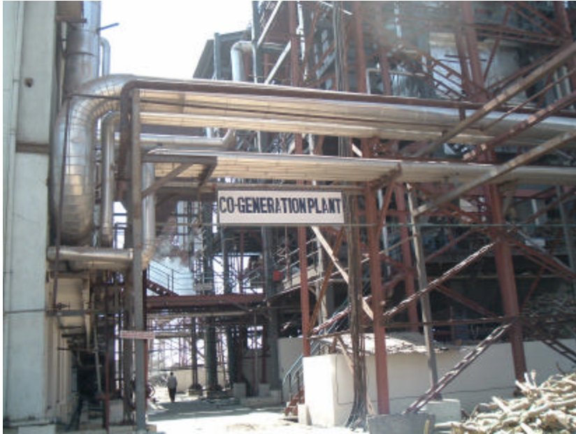
View of Cogeneration Plant in Sugar Mill
