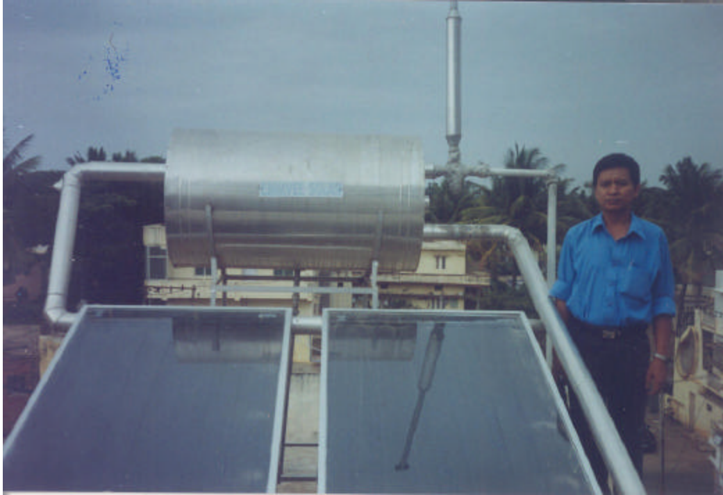
A Solar Thermal Unit – Domestic Premises
