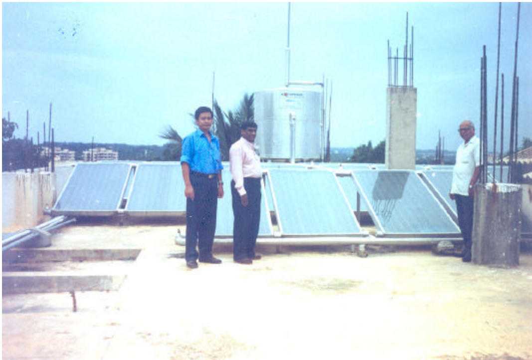
A Solar Thermal Unit – College Hostel
