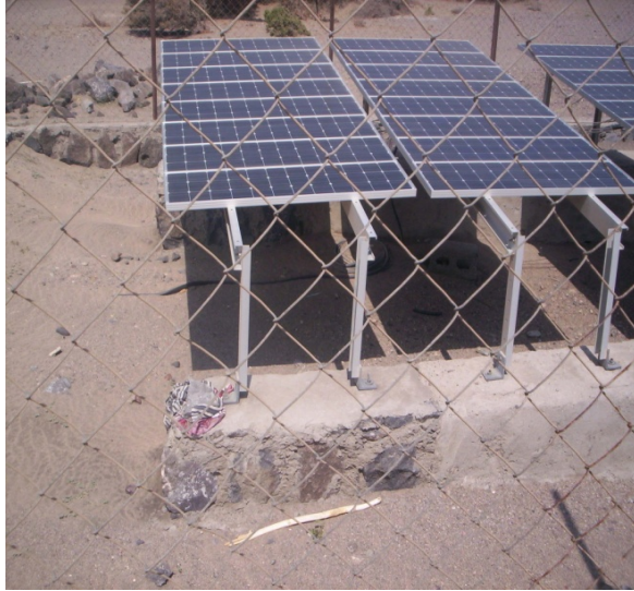
Photo: Solar System for Water Pumping – ERTC data has been instrumental in installation of solar for water pumping
