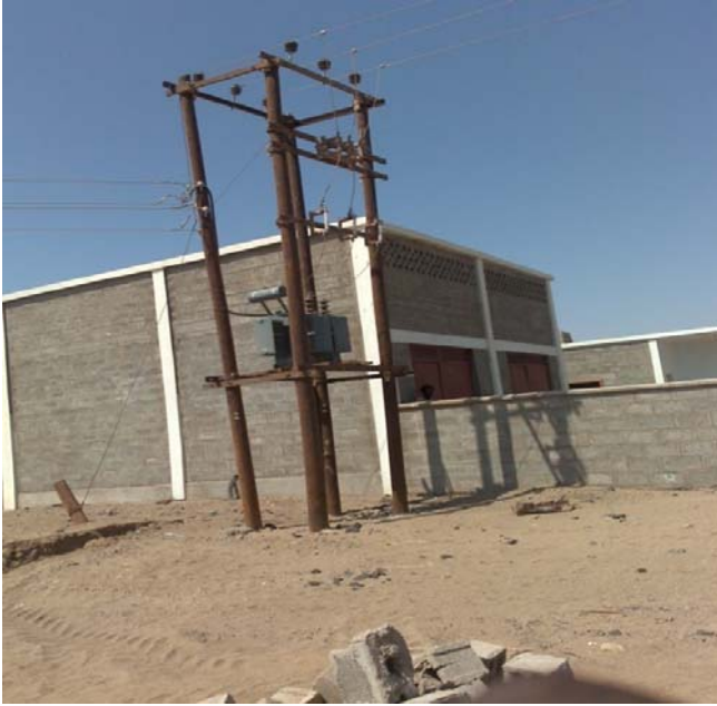
Photo: Completed powerhouse and grid reticulation at the project site
