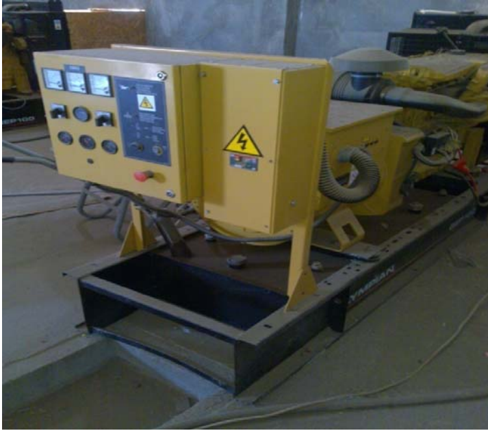
Photo: Diesel genset at Idi, which will operate in conjunction with wind, thereby reducing reliance on fossil fuel and enabling access to energy to this unelectrified village.
