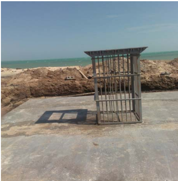
Photo: PMU modified platform design for the distributed wind system showing removal of redundant bars and the design of an elevated platform and widened foundation (to accommodate high water levels due to the proximity to the sea) accepted by contractor
