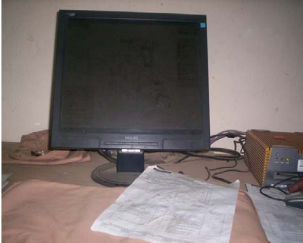
Photo: SCADA system installed at Assab wind farm for performance monitoring
